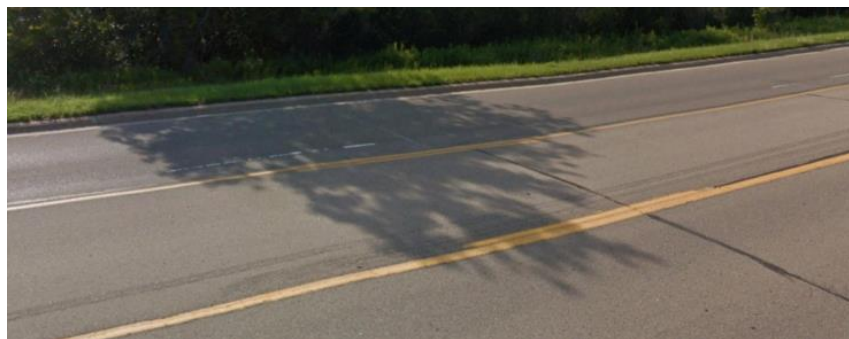
Figure 19: Conflicting Pavement Markings
